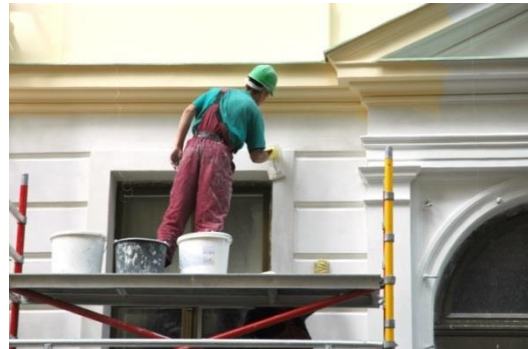
Maintenance- Preserving maintenance of buildings to protect life safety and to show someone cares about their property.
